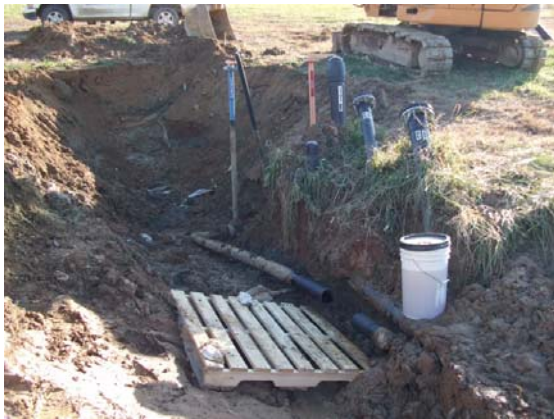
Hole in Pipe
